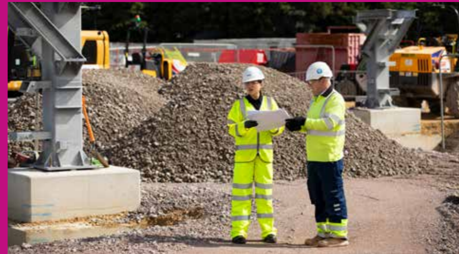
Learning by doing: Middlesbrough College's Maisy Macuzzi with Sofia's onshore converter station site manager Matthew Archer during her work placement with the project.
