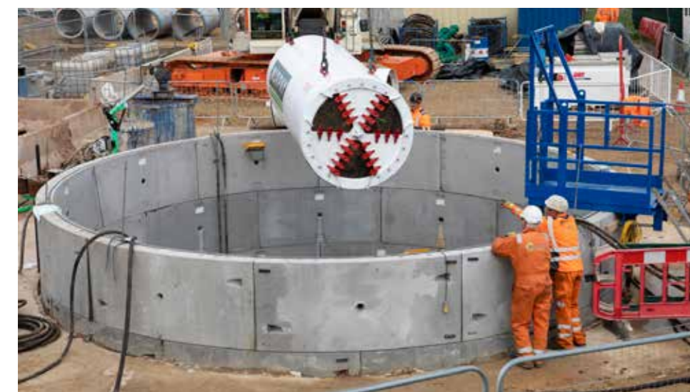
The tunnel boring machine being lowered into the shaft (Photo: Cal Carey)
